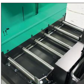
Battery on steel rollers
